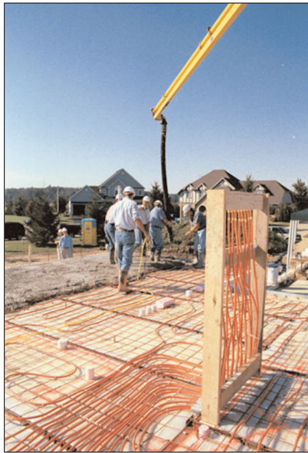
Figure 1. Hydronic radiant floor heating tubing laid out in specific heating pattern prior to concrete pour. Photo courtesy of Ready Mixed Concrete Association of Ontario.
