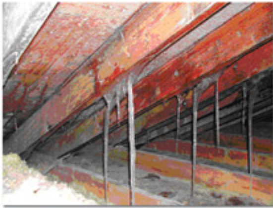
Condensation resulting from excess moisture being dumped into the attic has frozen on the underside of the roof sheathing.
