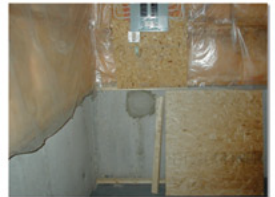
Notice the patched hole in the foundation below the electrical panel where stolen power was brought into the home.
